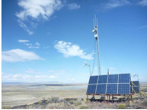
Figure 3.40: The Black Rock Mesa communication tower, one of three in the array. There are three stands each with solar panels. Those stands contain batteries, data acquisition PC and network instruments for long distance link.
